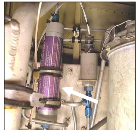
Emergency Brake System Accumulator
